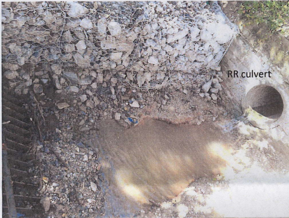
Improvements to pipe junction in August 2014 to aid maintenance and prevent pipe clogging.
